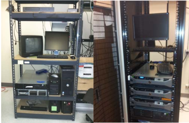
Servers consolidated into new machines and a new rack.
